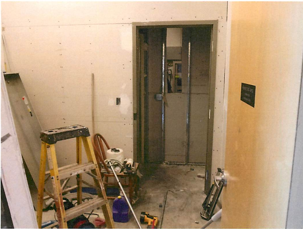
Data Closet Expansion – MDF, Redmond Building One
