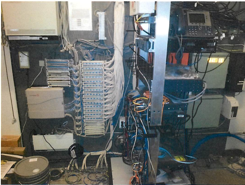
Existing Data Closet – IDF, Redmond Building One
