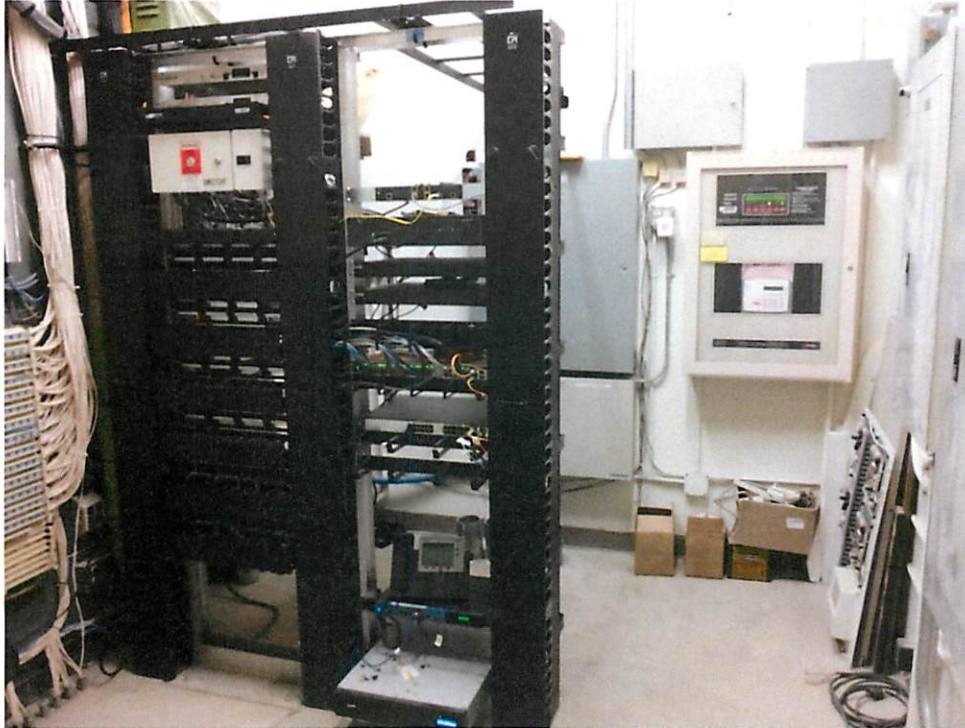
Data Closet Expansion – MDF, Redmond Building One
