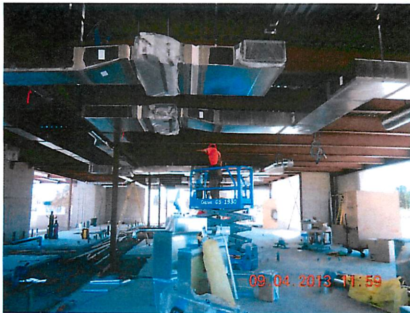
Ductwork on the 1 st floor South Wing
