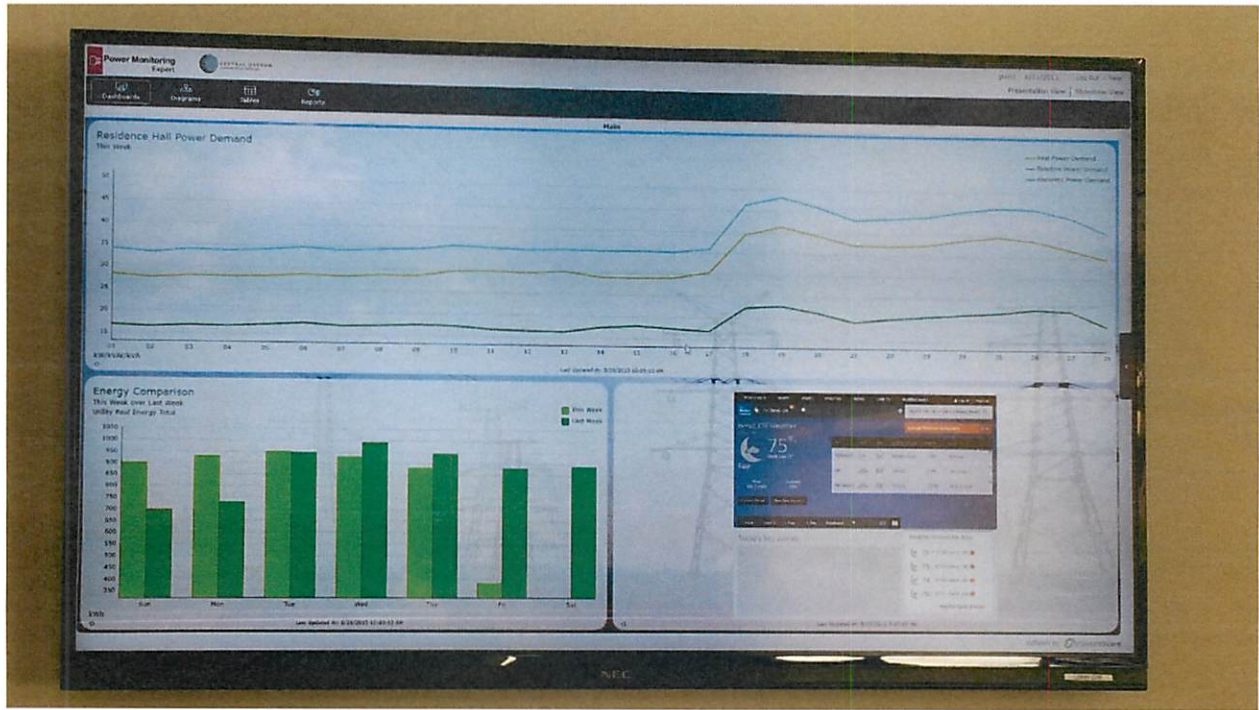
Power Monitoring Software Installation – Lobby Display.
