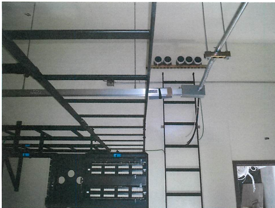
Infrastructure prior to data installation – South Wall, MDF
