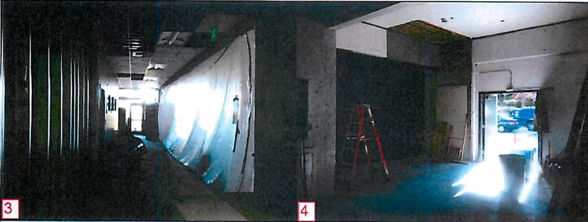
3 Asbestos abatement in N/S Sisters classrooms. 4 Old loading zone to become offices.
