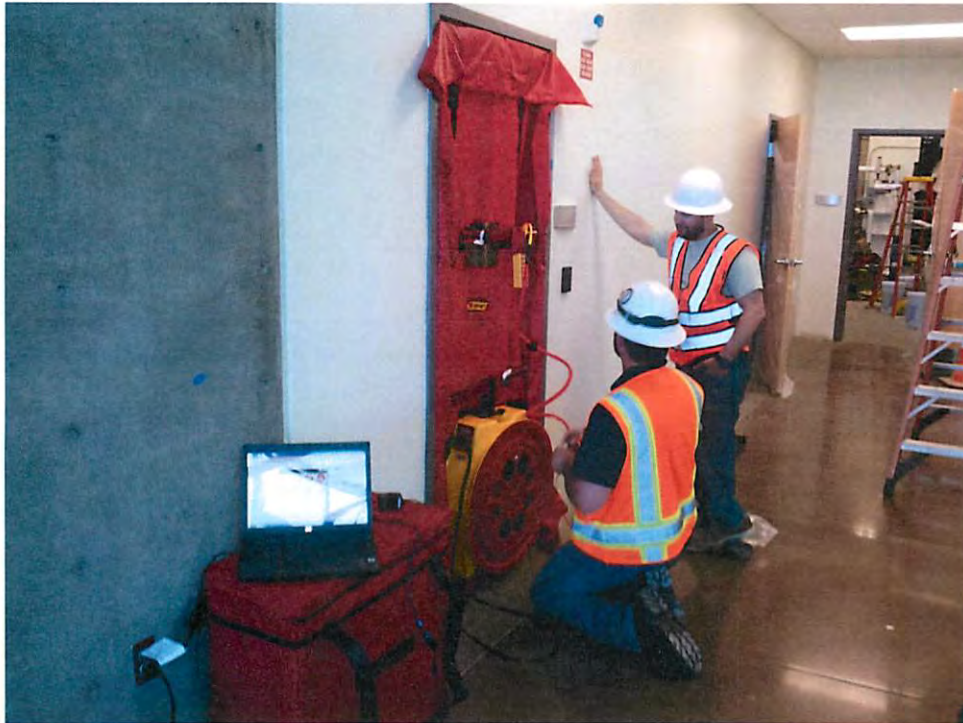
Chemical Fire Suppression Testing –MDF, 2 nd Floor
