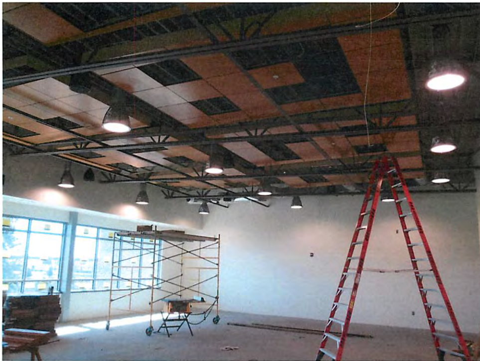
Speaker Installations – Community Room
