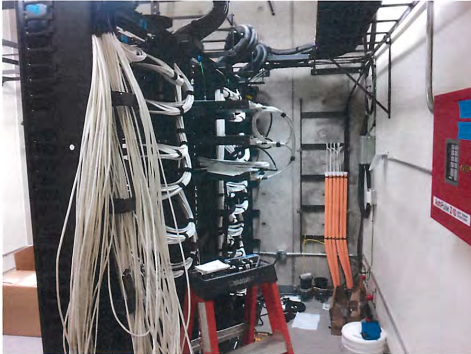
Data Cable Terminations – MDF 209
