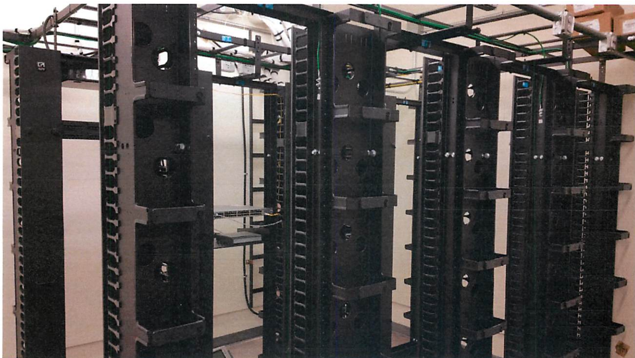
Network Rack Installation – Residence Hall, MDF
