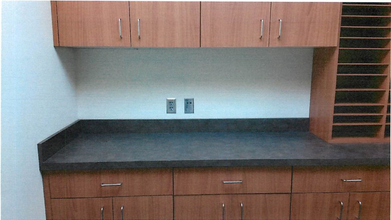
Power and Data – Ochoco, Workroom
