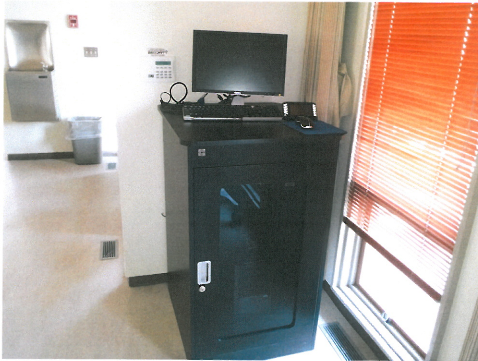
Audio-Visual Cabinet – Chandler Building, Meeting Room 301
