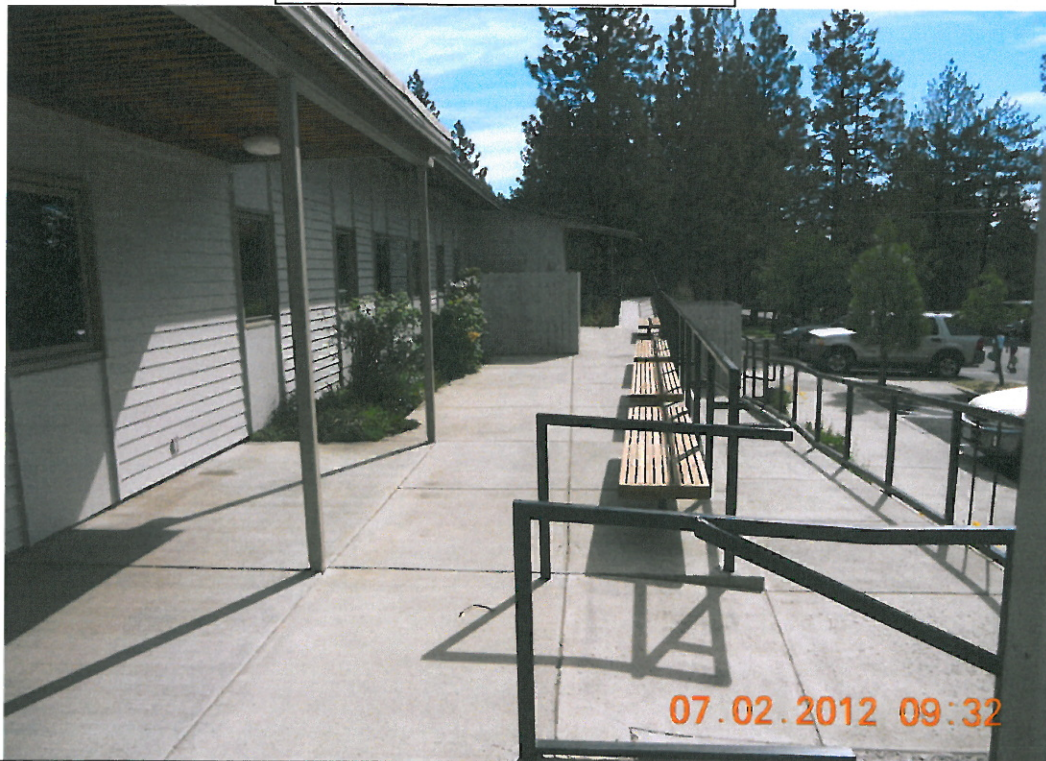
Entry ramp work and landscape complete. Railing painted and benches cleaned and sealed.
