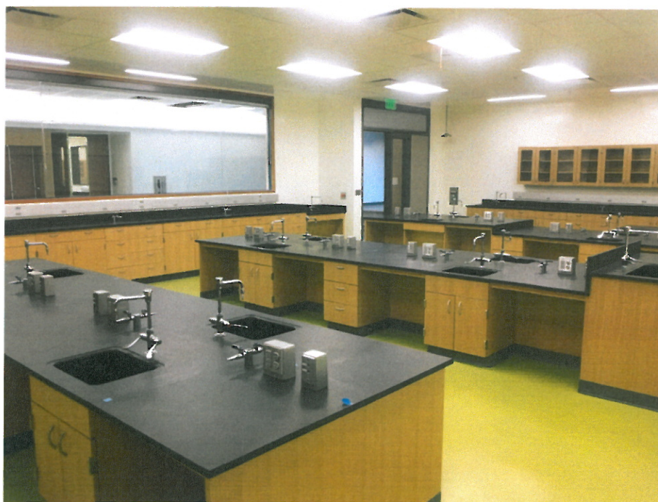
Above Counter Data Ports – Science Building, Lab 140
