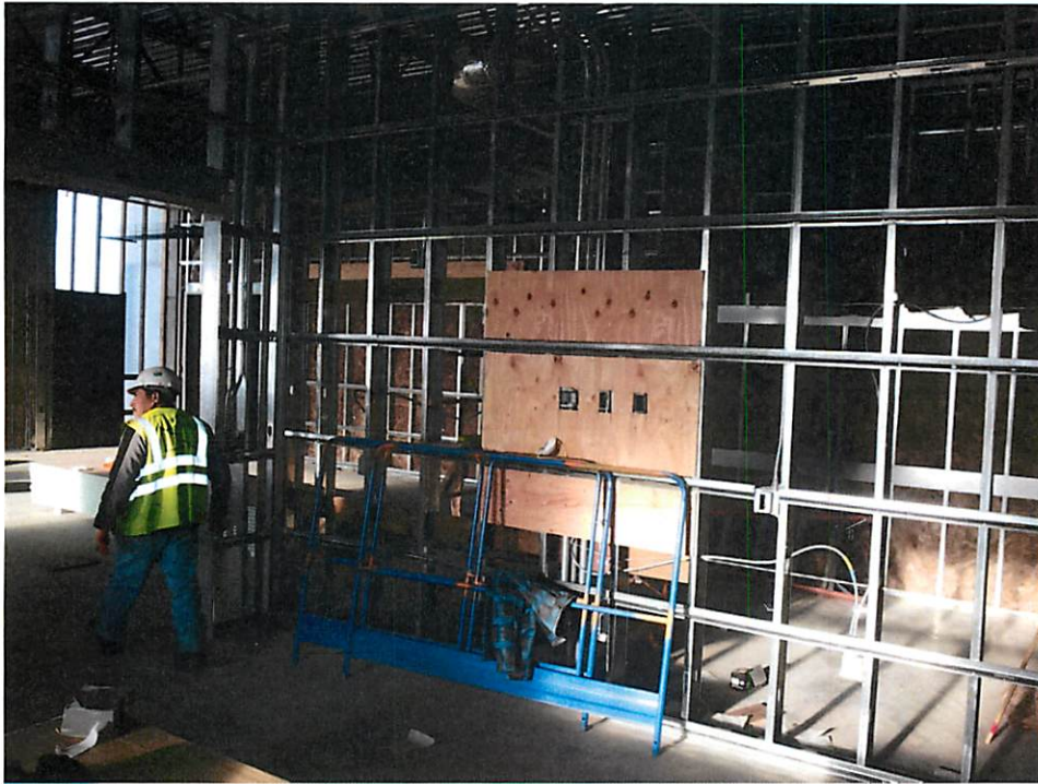
LCD Backing & Backboxes – Conference Room 222, 2 nd floor
