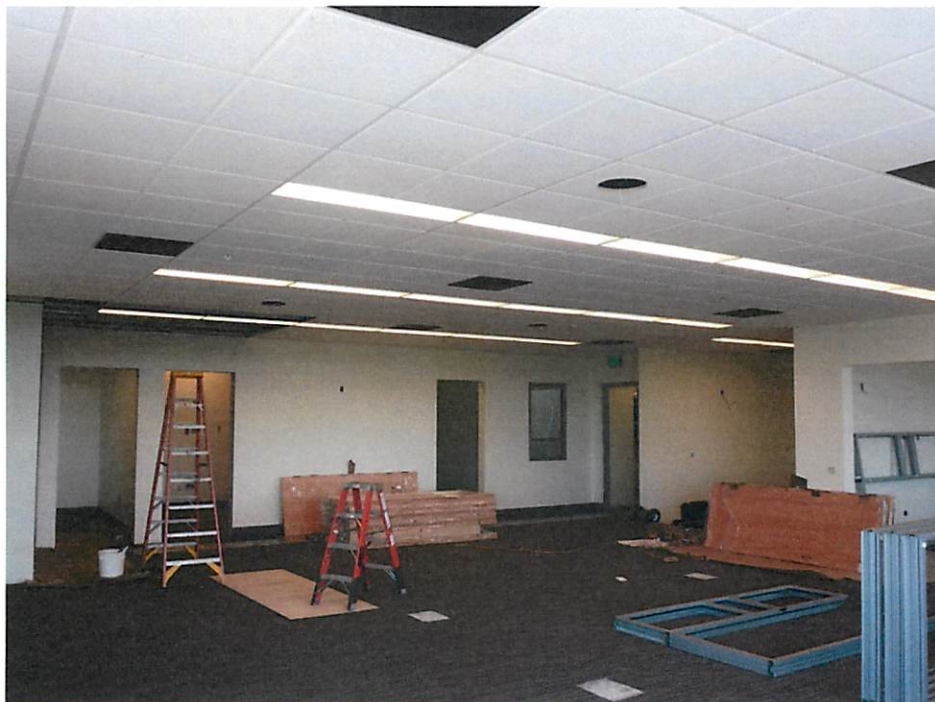
Projection Wall & Speaker Tiles – CEED 223
