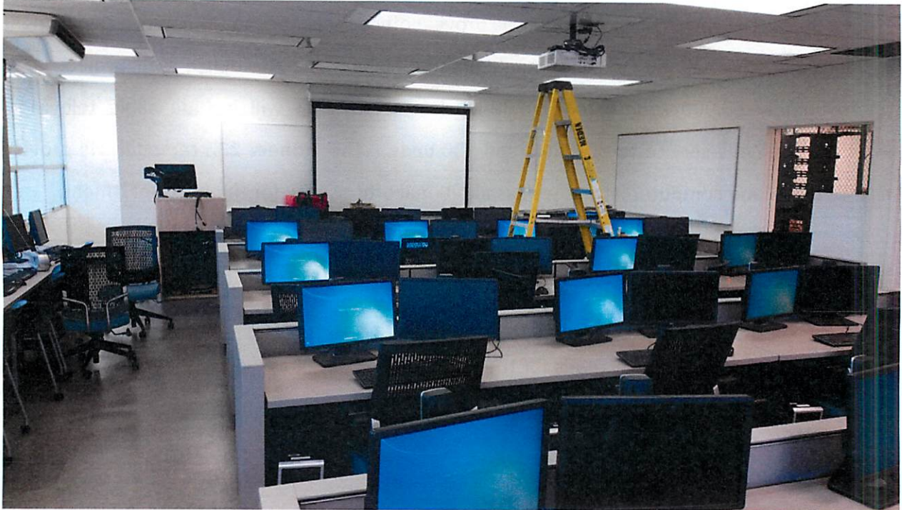
Speaker, Projector and PC Installations by COCC IT Staff in Progress – Pioneer 232
