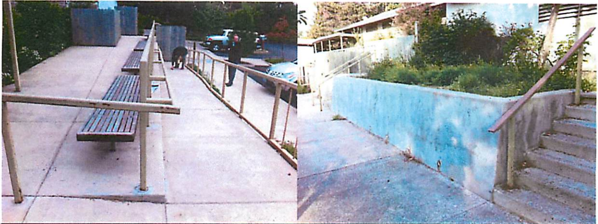
Entry ramp to be repaired/reworked to provide ADA access to the front door.
