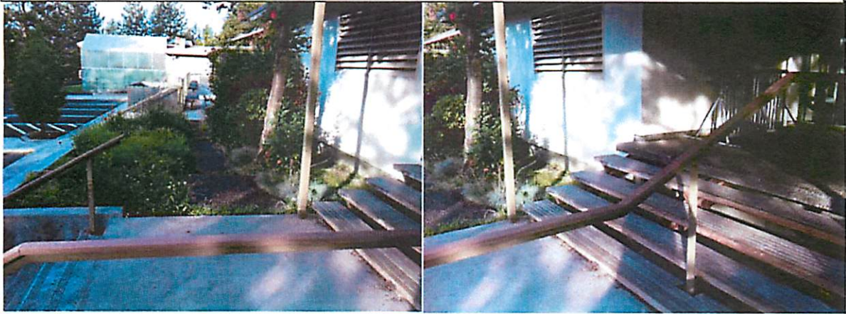
Intermediate landing and upper stairs at entry to be revised for ADA ramping.
